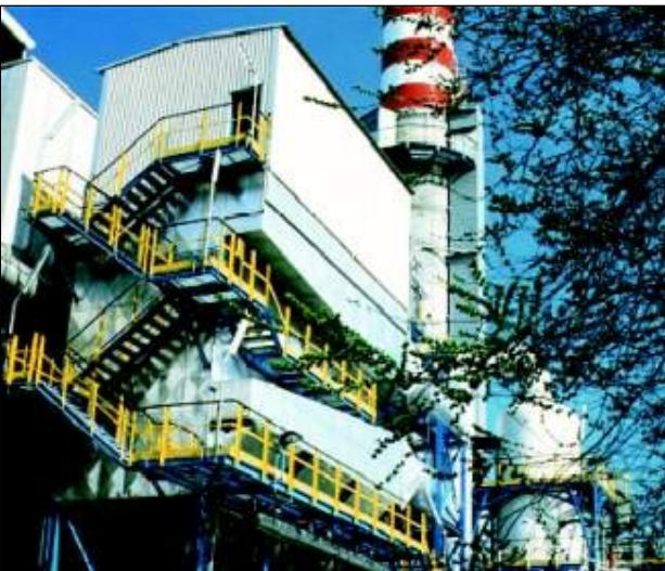
Municipal Solid Waste Incineration 16 MW – 65,000 ACFM
