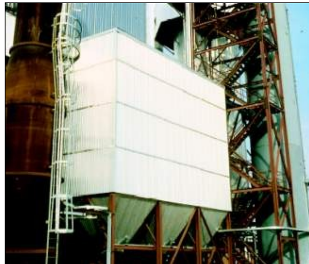
Coal-fired Industrial Boiler 110,000 ACFM
